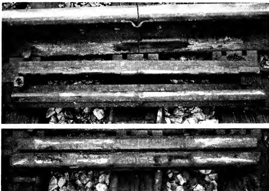
Fig. 6. North Portion Section 2, Conoco Anti-Rust Compound (Brush coat on rail and bars)
